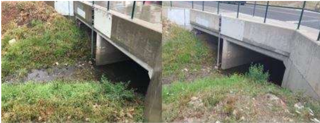
Figure 1-4 - Knoles Drive culvert with water flowing (left) and water pooled (right)
