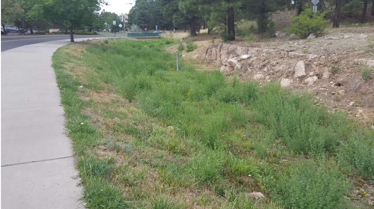
Figure 1-3 - Overgrown vegetation in portion of Sinclair Wash
